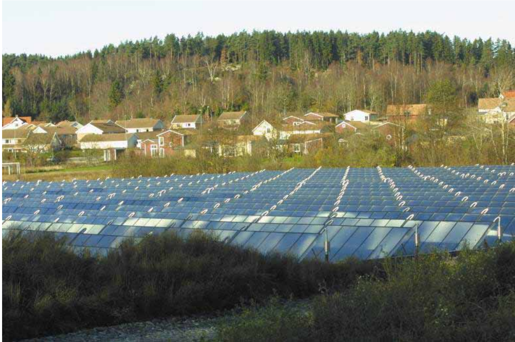
Solar plant combined with district heating, 10.000 m 2 , Kungälv Sweden Source: ARCON / ESTIF
